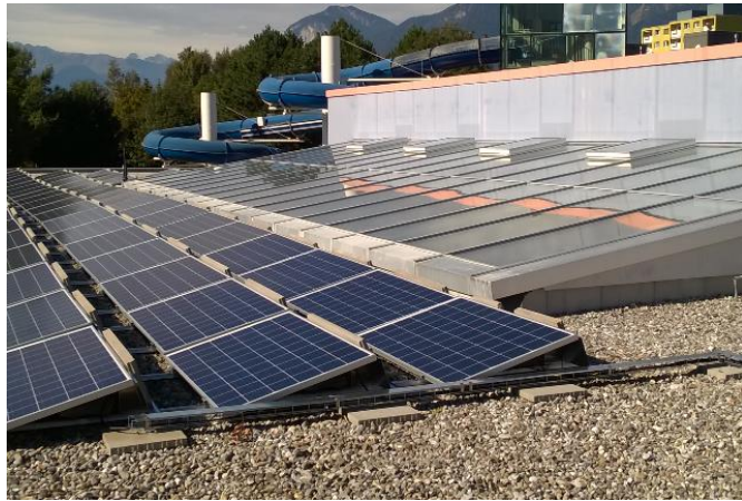
Figure 3: PV plant at public indoor swimming pool
