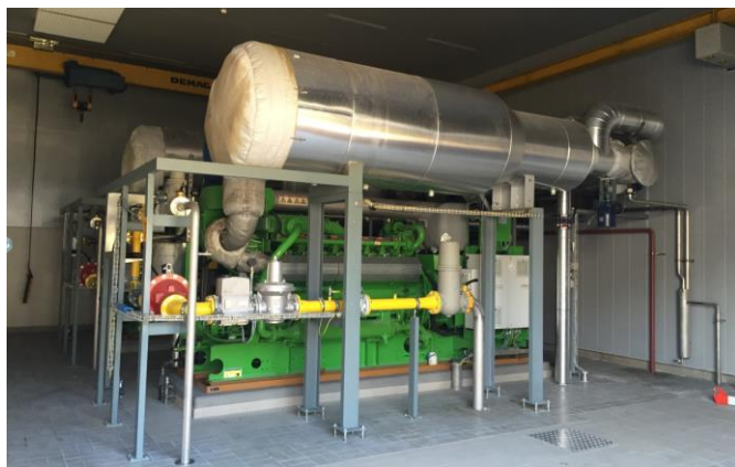
Figure 4: biogas CHP at the side of WWTP
