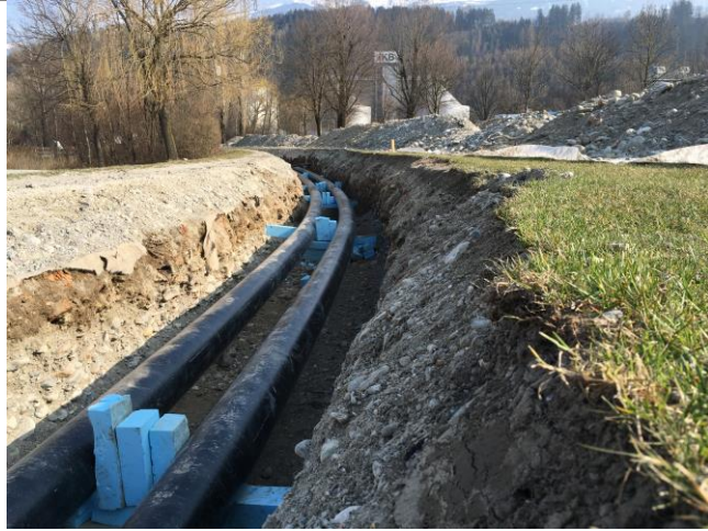
Figure 2: district heating pipes from WWTP to public indoor swimming pool
