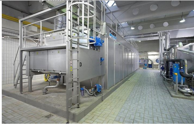
Figure 5: sewage sludge dryer at the side of WWTP
